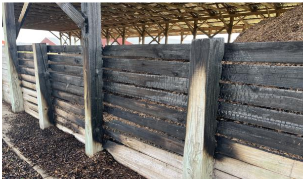
Figure 2. Litter overheated and caught this stacking shed sidewall on fire.
