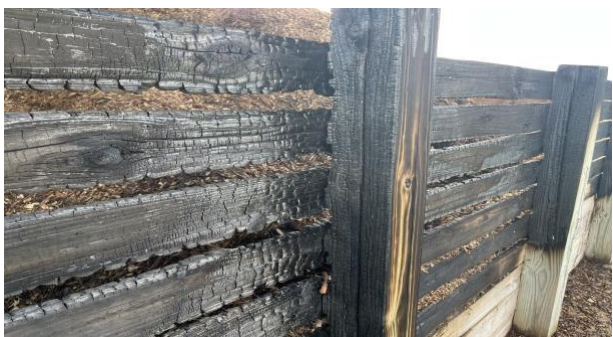
Figure 4. Lumber and posts destroyed by overheated litter in a stacking shed.
