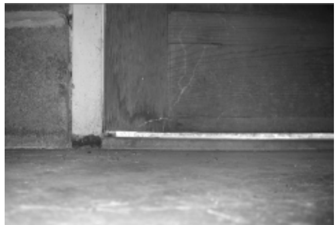
Gaps around doors should be sealed.
