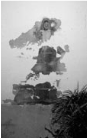
Repair plumbing leaks as quickly as possible. Moisture attracts termites to the structure.
